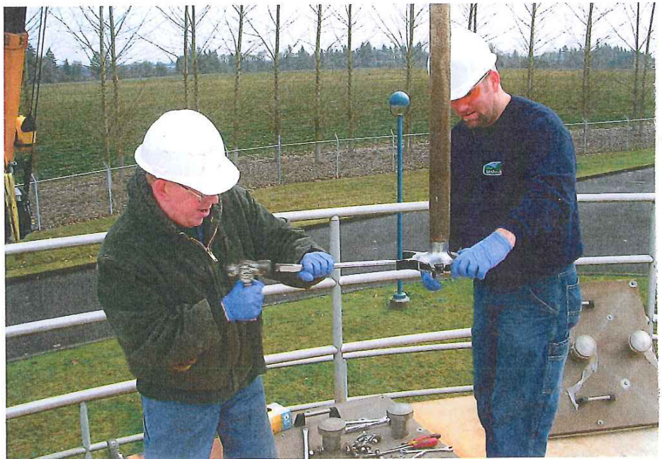
Lee Koester and Roy Carter work on an additional aerator that was added to the facility's digesters to increase capacity. David Gehring
