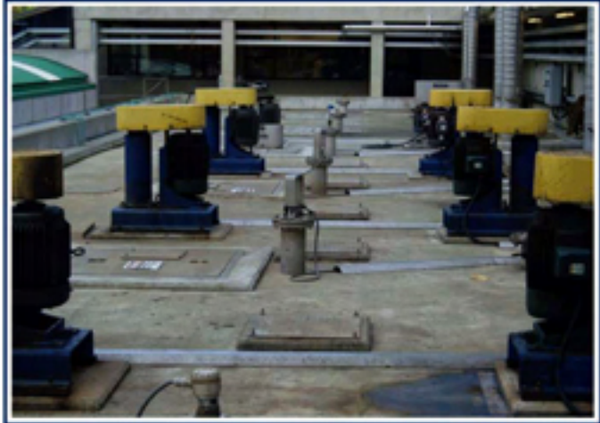
ATAD Installation – Canada
