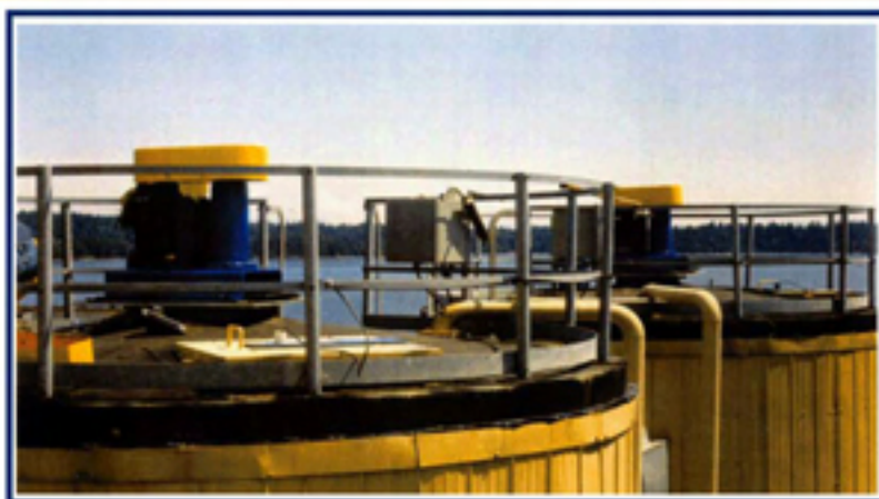
ATAD Installation – Canada
